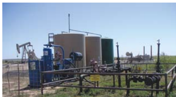
Ellis-2 Site Facilities.
